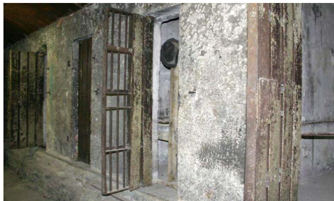
Jail cells that were used to hold inmates during territorial days remain intact in the basement of the Crawford County Courthouse after a recent courthouse remodeling project. Informal jail tours in an area known as “the dungeon” have become popular, especially on Halloween.
